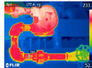
Below: Replacement steam trap operating properly (note condensate return temperature now 177.4°F)
