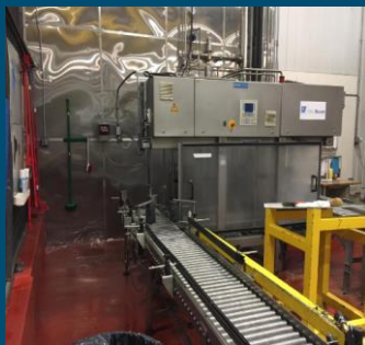
Keg washer, Draining Steam Condensate
